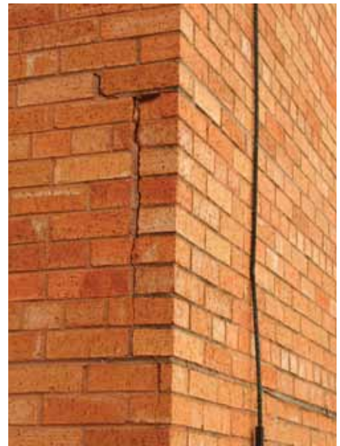
Cracked corner brick resulting from a lack of expansion joints in the brick veneer.
