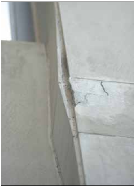
Failure of relief angles above causes limestone curtainwall to buckle under the panel weight from above.
