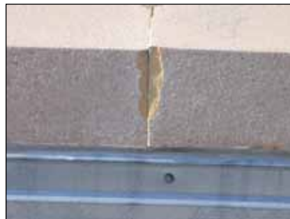
Mortar joints that are too small can cause spalls when terra cotta coping expands.
