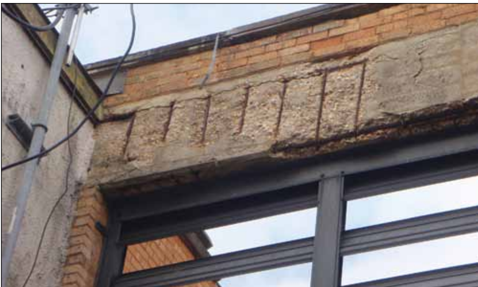
Corrosion of the reinforcing steel has caused the concrete cover to spall.
