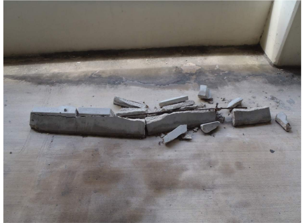
Broken Wheel Stop
