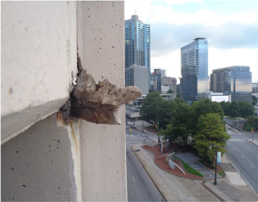
Spall Over Sidewalk
