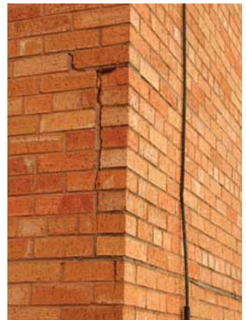
Cracked corner brick resulting from a lack of expansion joints in the brick veneer.
