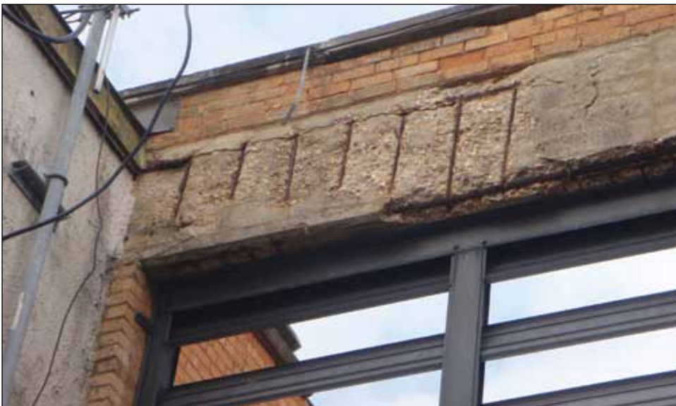
Corrosion of the reinforcing steel has caused the concrete cover to spall.
