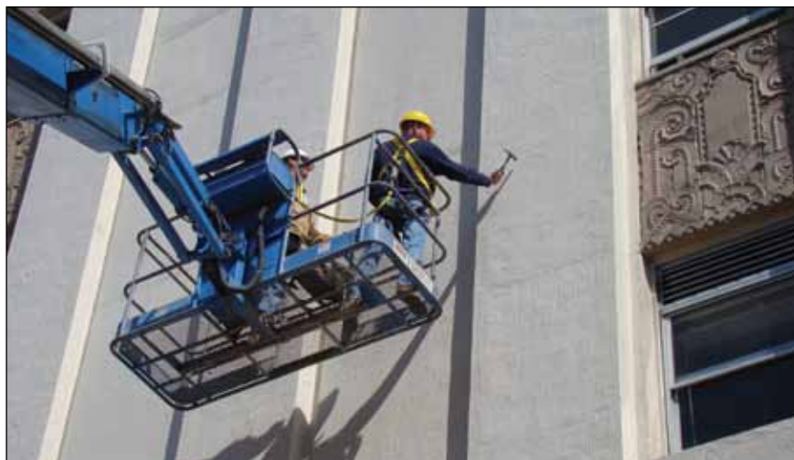
Detailed Façade inspection including sounding for delamination being conducted from a telescoping boom lift.
