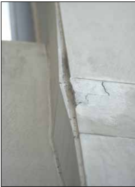
Failure of relief angles above causes limestone curtainwall to buckle under the panel weight from above.
