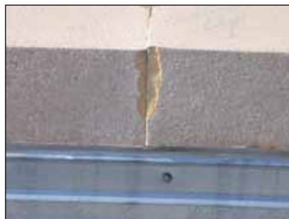
Mortar joints that are too small can cause spalls when terra cotta coping expands.
